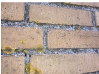
Fine vandrette revner i sten.
